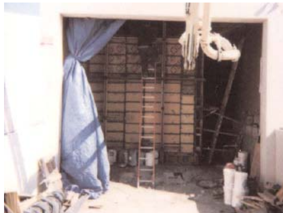
Difficult concrete pumping and building requirements for the indoor structure. KIM in the mix facilitates this unique design option.
